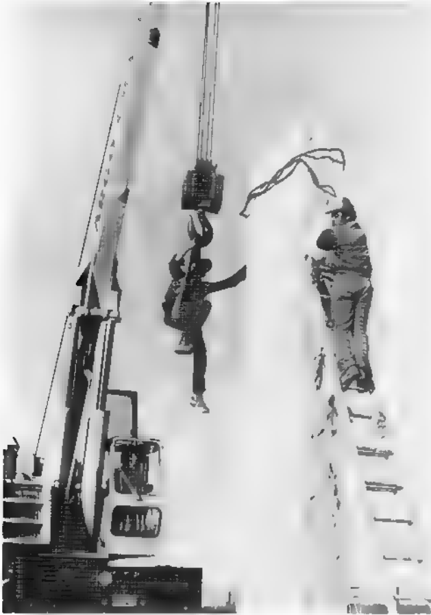
Workmen take cables loose as one of the Guidestones is placed in its rightful position. The rock-pitched finish on the sides is in accordance with "Mr. R.C. Christians'" instructions, that the finish conform as nearly as possible to the natural state of the granite as it is quarried.
